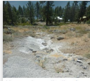
Heavy channelization from I-80, looking downhill.
