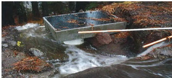
Utilities connecting West Donner to East Donner and located along Reed Avenue West compromised by runoff.
